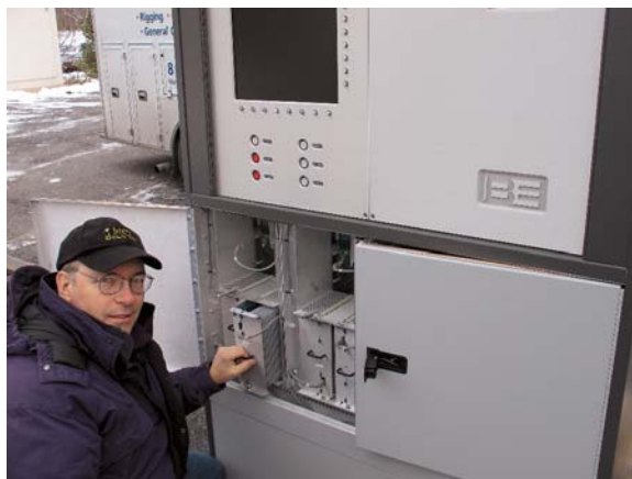
Loud & Clean's John Garrett tags and removes all the RF Power Supply and PA modules to lighten the 4MX 50 cabinet for insertion into the room.
